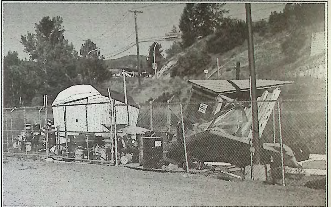
These two storage sheds, located at the Esso Cardlock on Burton Avenue, were severely damaged by what eyewitnesses called a tornado. A 'swirling cloud of brown dust' travelled down the Trans-Canada Trail late Friday afternoon then hit these sheds, which sit next to the railway right-of-way. The force of the disturbance blew part of the roof of the wooden structure 30 metres away.
