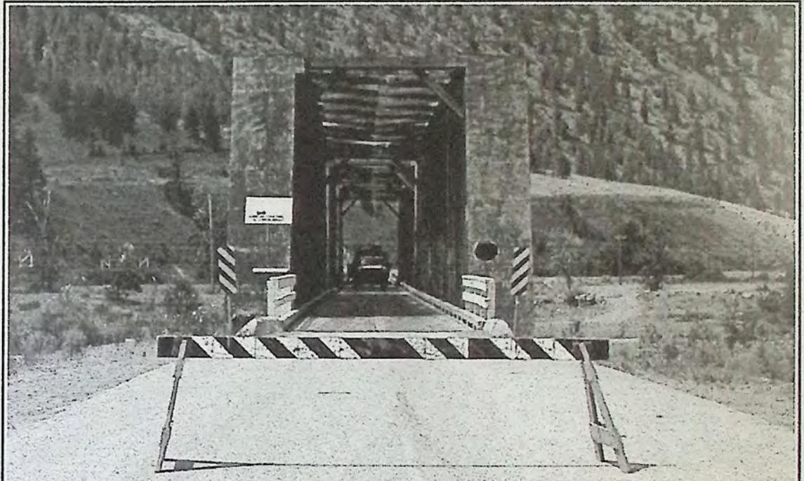
The historic red bridge in Keremeos is currently closed to all traffic. A major construction project will see the deck repaired and all siding replaced and repainted.
