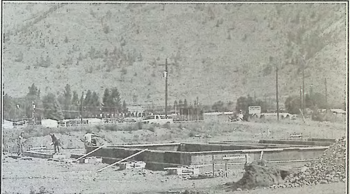
The foundation for the new RCMP station has been built. Wagers on who will serve in the building may become one of the key local entertainments.
