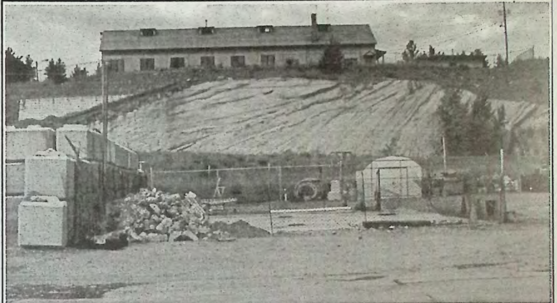
Work continued last week at the Esso Cardlock on Burton Avenue, owned and operated by Cool Creek Agencies. A new electronic metering system is being installed to allow operators of the cardlock system to read fuel levels in the underground tanks without having to open them. Photo above shows the diesel tank location of the lot partway through the installation phase.
