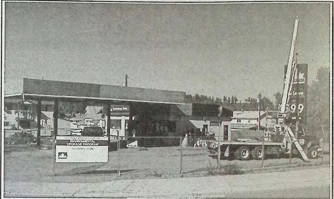
This was the scene last week as construction crews started working at the PetroCan station at the corner of Highway 3 and Bridge Street. In a few weeks the site will have a complete face lift.
