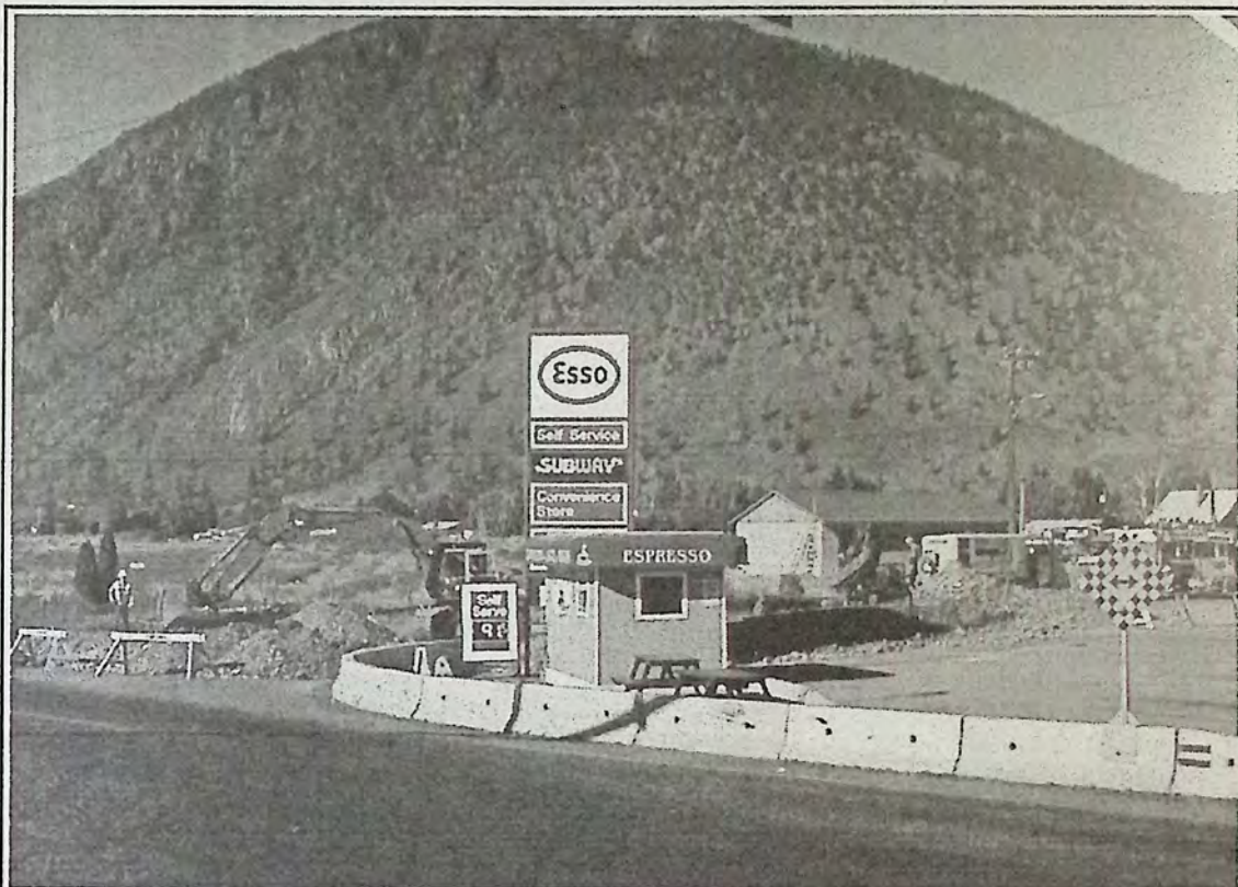
The Keremeos sewer system is being extended. Work began recently at the intersection of Highways 3 and 3A to provide service to Keremeos residents on the bench overlooking downtown.
