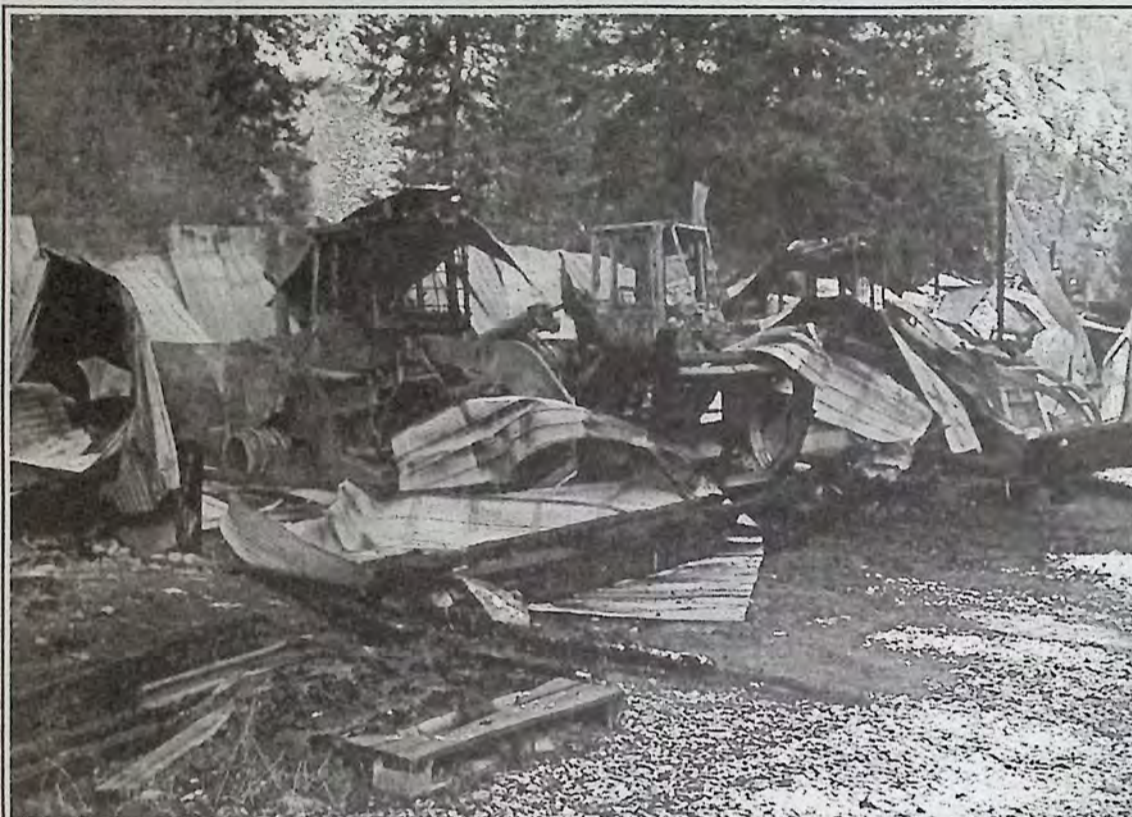
Princeton RCMP responded to a building fire at Princeton Wood Preservers Ltd. early the morning of December 8th. Upon arriving at the scene on Highway 3, about 18-km East of Princeton, Police and Fire Crews found the main shop (south of the office) fully engulfed in flames. The cause of the fire is still unknown. There was extensive damage to the building and equipment being housed inside. Photo: Brenda Engel.
