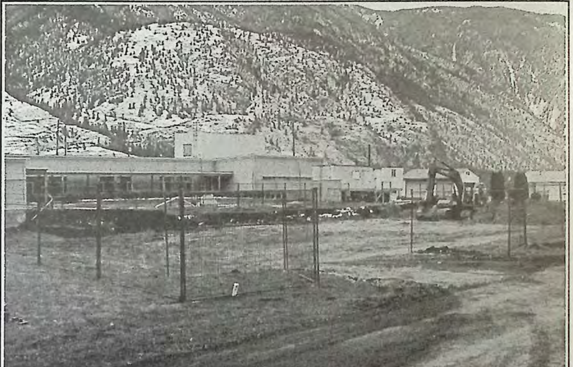
Site prep continues on the Assisted Living project located next to the Keremeos Health Centre.
