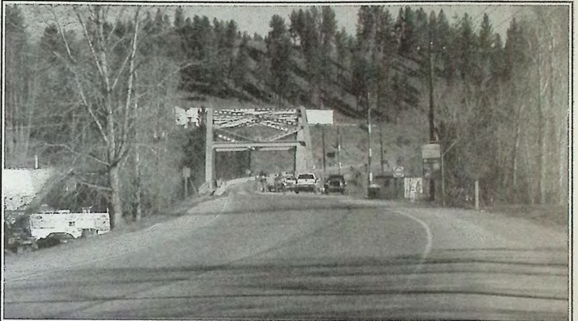
Local traffic has been limited to one lane on the steel bridge over Tulameen River on Highway 5A while crews repaired the bridge surface last week.
