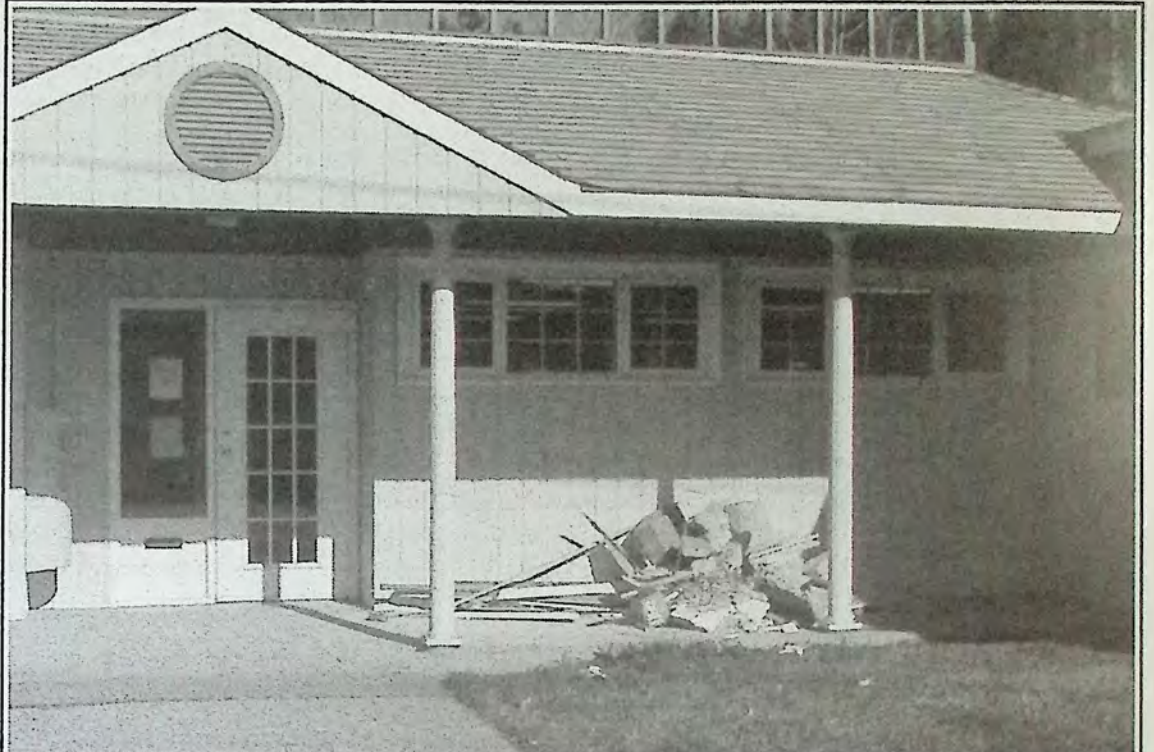
Renovations are underway in the former Public Health Unit building. The Town of Princeton has leased it to Princeton & District Community Services Society. The New Beginnings program and the administration offices will move to the new location. New Beginnings has been in the Elks Hall for a number of years, and the administration offices have been located in a large heritage home on Halliford Avenue.
