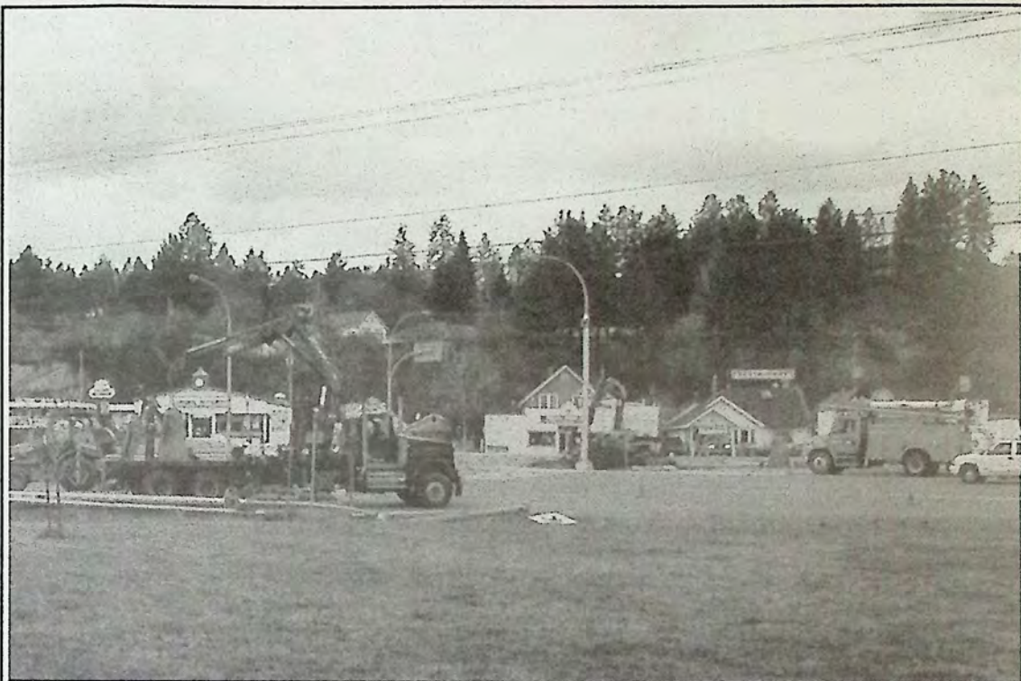
Highways crews worked for most of the day last Tuesday installing the new pedestrian-controlled crossing signal at Highway 3 and Burton Avenue. The signal was completely installed by the next day.
