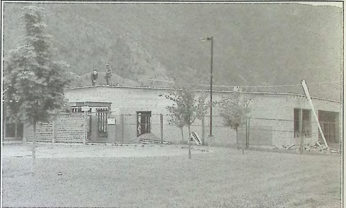
Construction is progressing well on the Assisted Living Complex in Keremeos. Eileen Oliver-Bauer of Lower Similkameen Community Services Society says the roof went up last week. The project is expected to be complete in October with the first residents to move in by mid-November. "Everything is on time at this time," Oliver-Bauer says.
