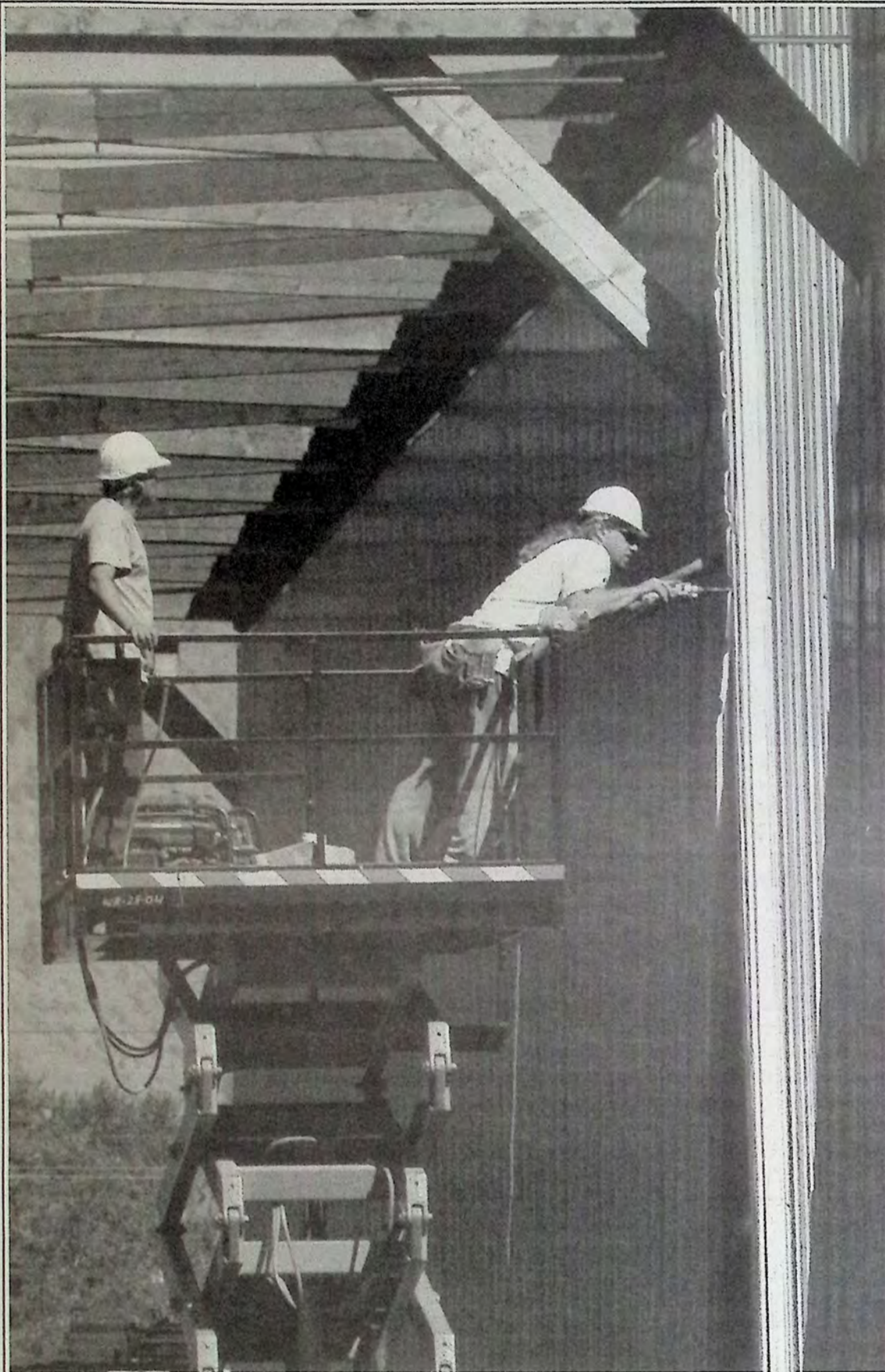
This bridge crew was captured working hard last week on the inside panels of the historic Red Bridge in Keremeos. Photo: Bryan Smith, www.keremeos.net.
