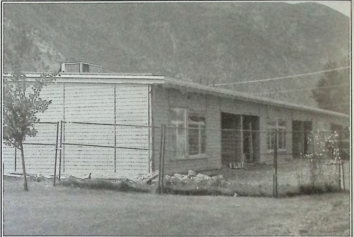
Progress continues to be made on the Assisted Living Complex in Keremeos.
