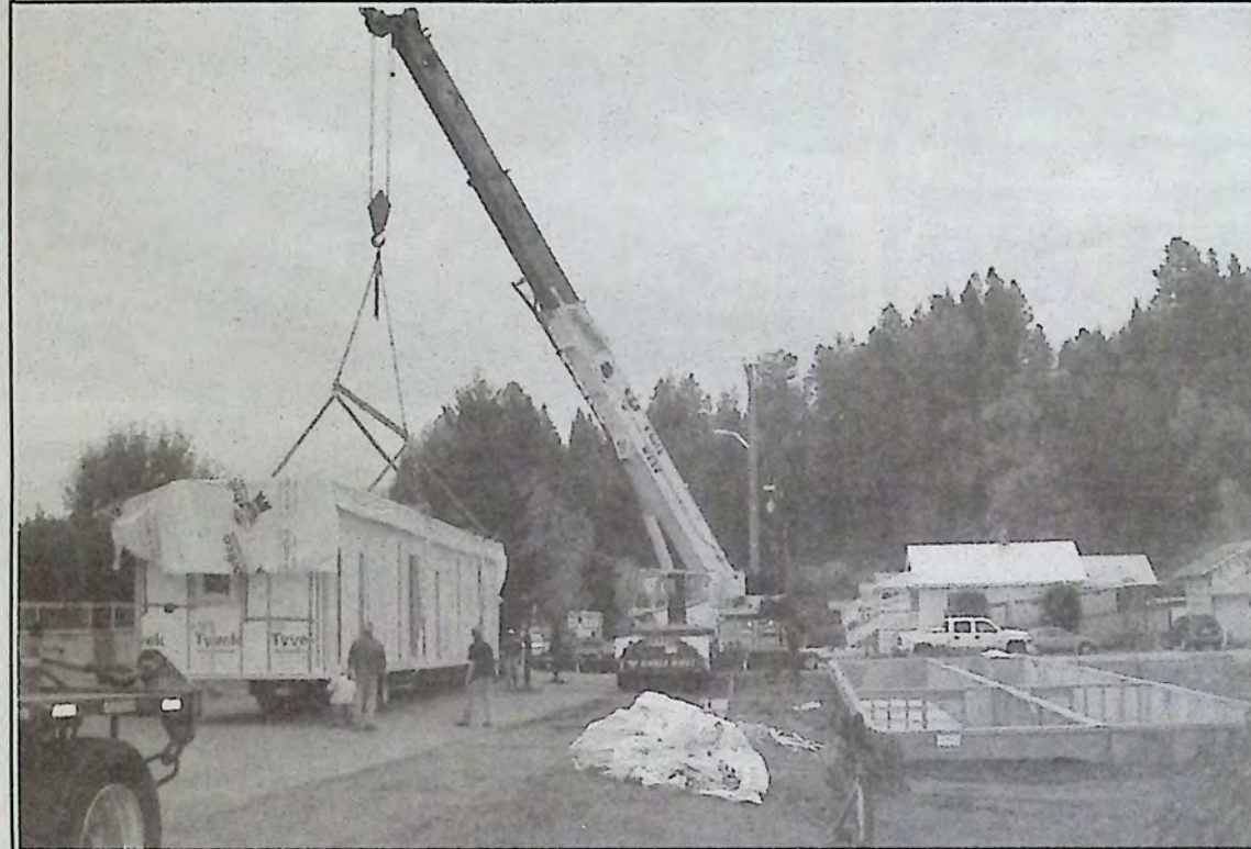
Activity in the Allison Flats neighbourhood has never been like this! Heavy equipment moved parts of the new Mary Anne Apartments in place all week long. This section was placed Wednesday.
