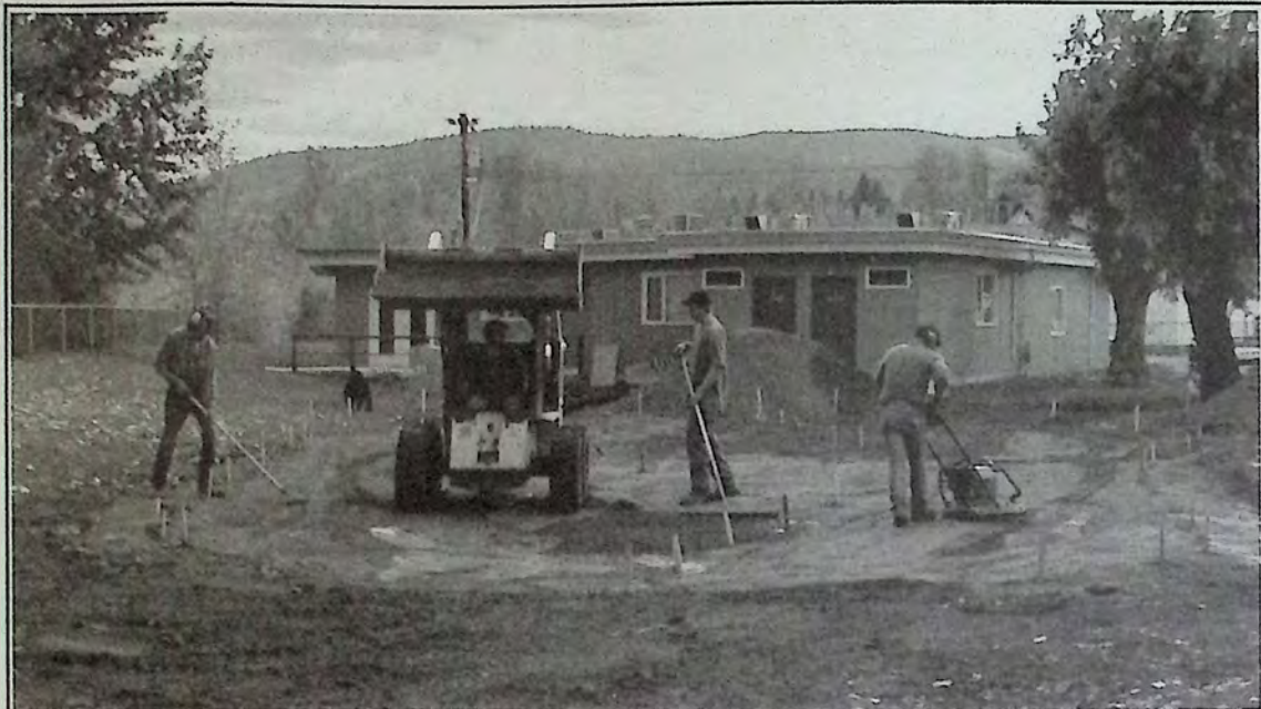
Splash Park, anyone? Work progressed well last week in Rotary Park on the new Splash Park.
