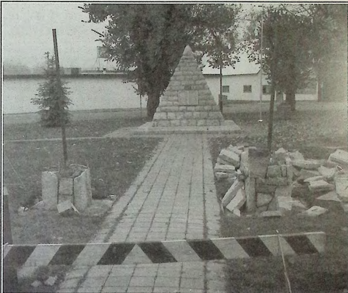
Here's another look at the progress being made on the new arch at Cenotaph Park. This photo, taken early Saturday morning, shows a little more of the detail rock work going into the project.
