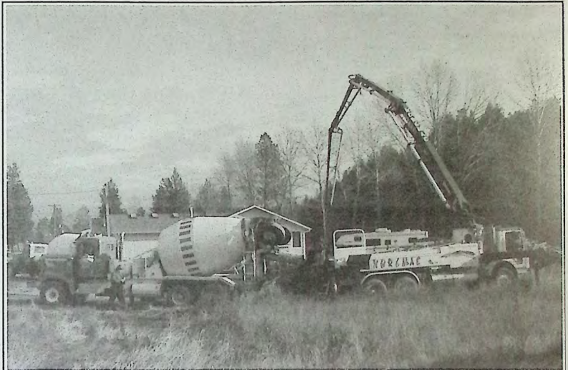
Foundation pouring with a crane truck became a spectator sport for many last Friday on Corina Avenue. It's a sure sign of development of riverfront property!
