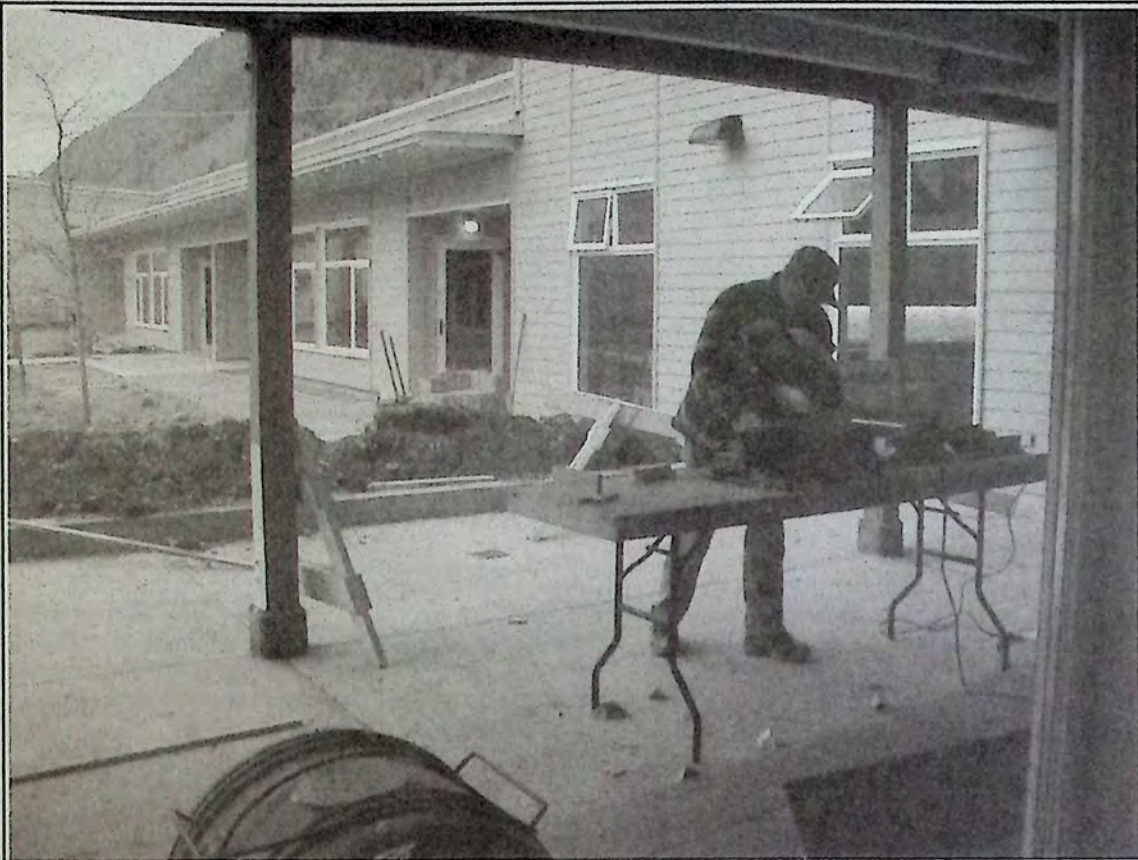
The finishing touches were being put in place last week at the assisted living wing at Keremeos Health Centre. The facility has already had some residents move in.
