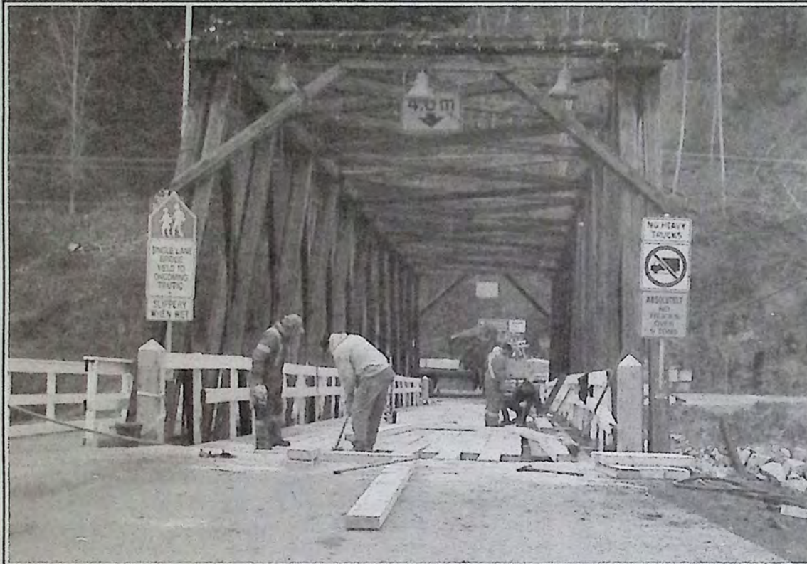
The wooden bridge at the end of Bridge Street was closed for part of last week to allow crews time to replace planks in the bridge decking. Traffic was re-routed around town over the Silver Bridge.
