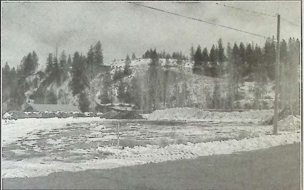
This collection of lots at the corner of Waterfront Avenue and Bar Street were cleared last week to prepare them for construction. Some of the lots face the Similkameen River.
