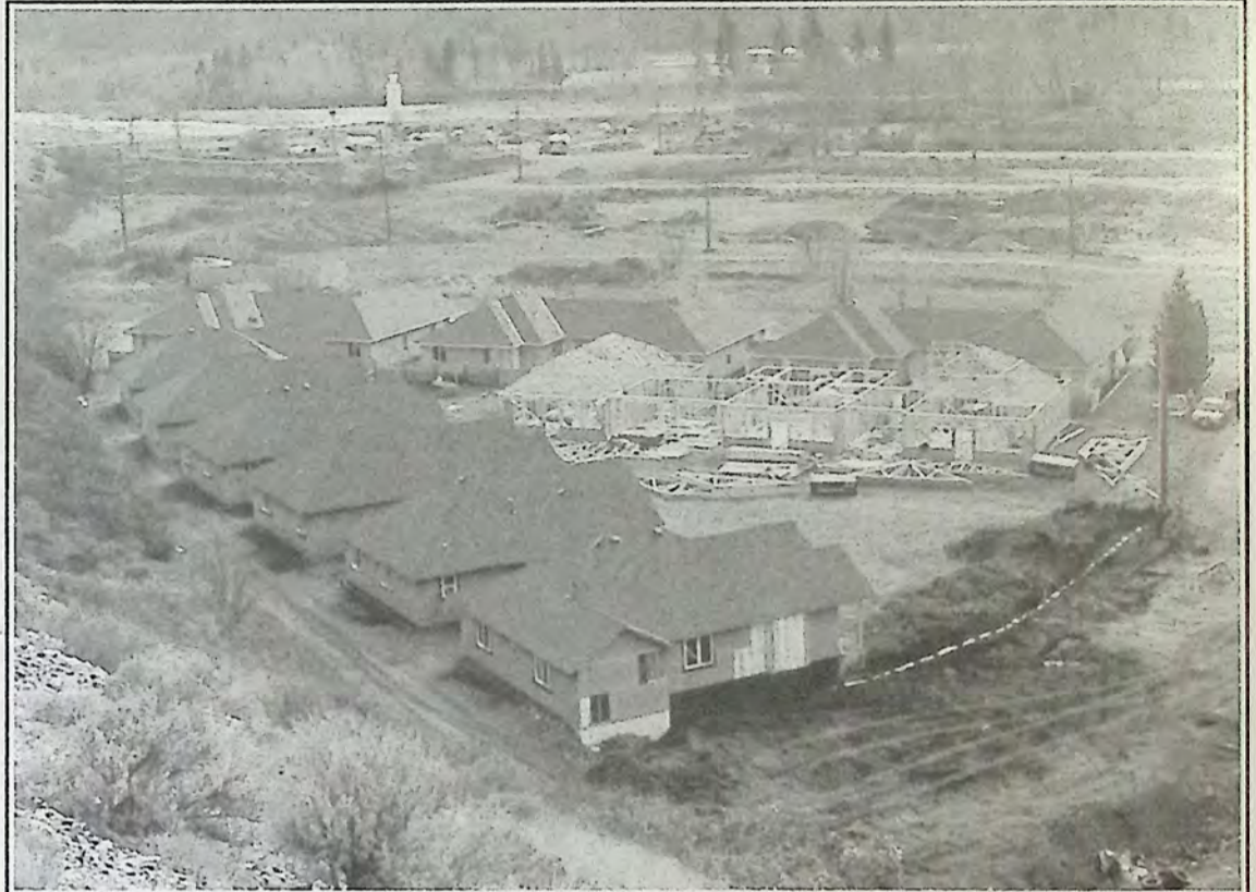
Construction continues as Keremeos experiences a small growth spurt. This subdivision is located just below the RCMP Station at the end of Sixth Avenue.
