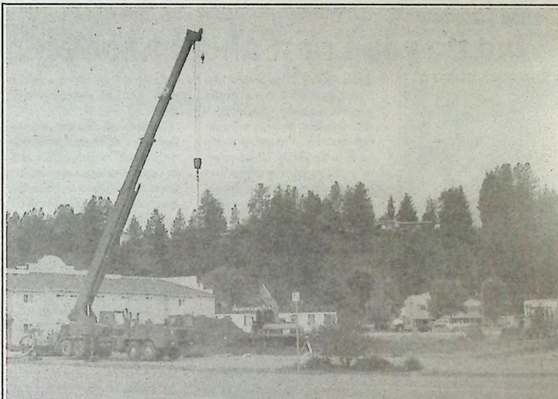
Construction continues on Highway 3 between Best Western and Dairy Queen on the new gas station/doughnut shop - one of many new developments in and around Princeton.
