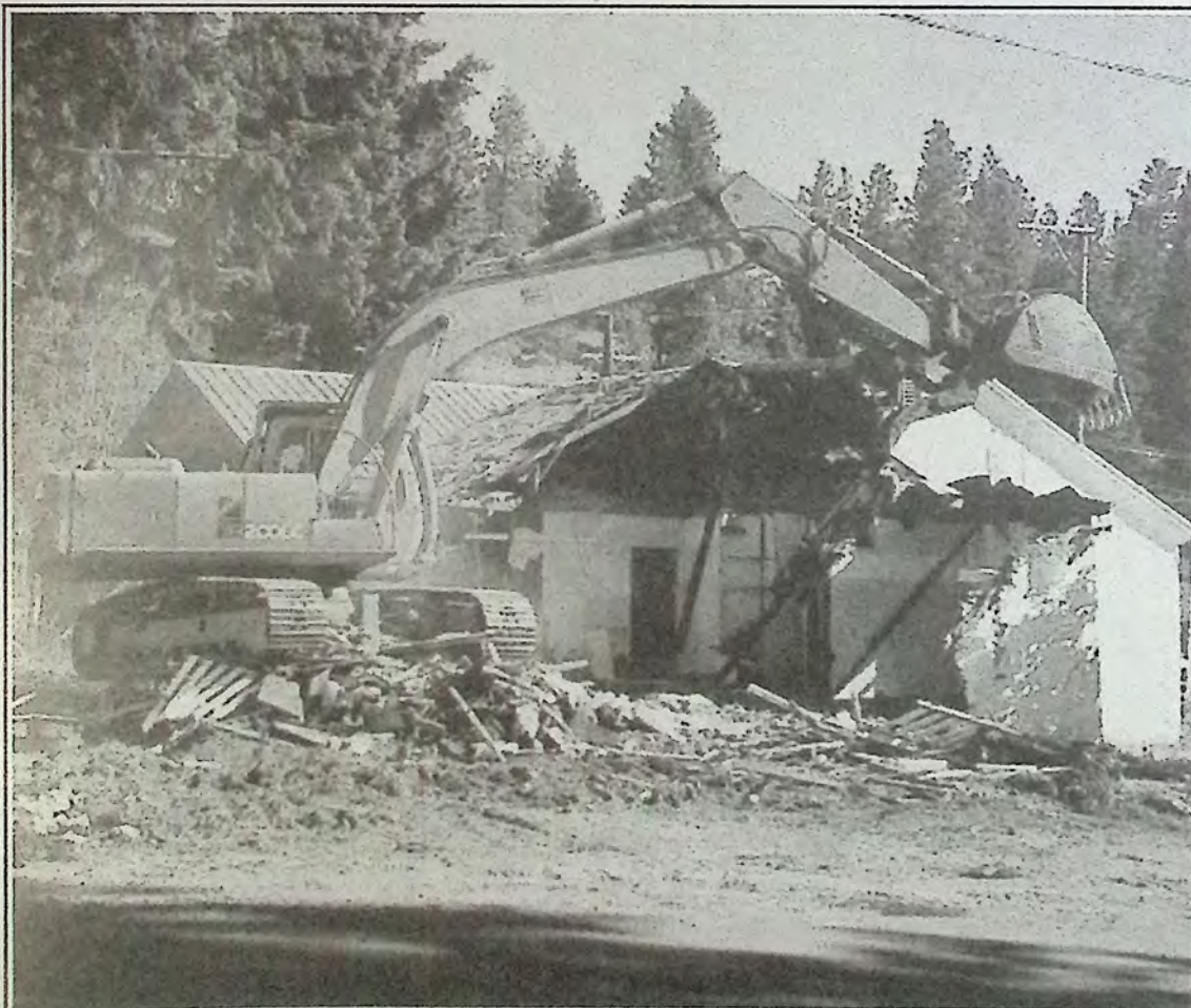
Now you don't...The view part way through demolition on July 17th. Photo: Norm McGivern
