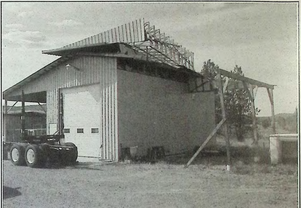
A mini 'twister' cut through property along Princeton-Summerland Highway at about 1:00 PM last Tuesday. It flipped this roof over near Sunflower Downs and tore off shingles from another nearby building.
