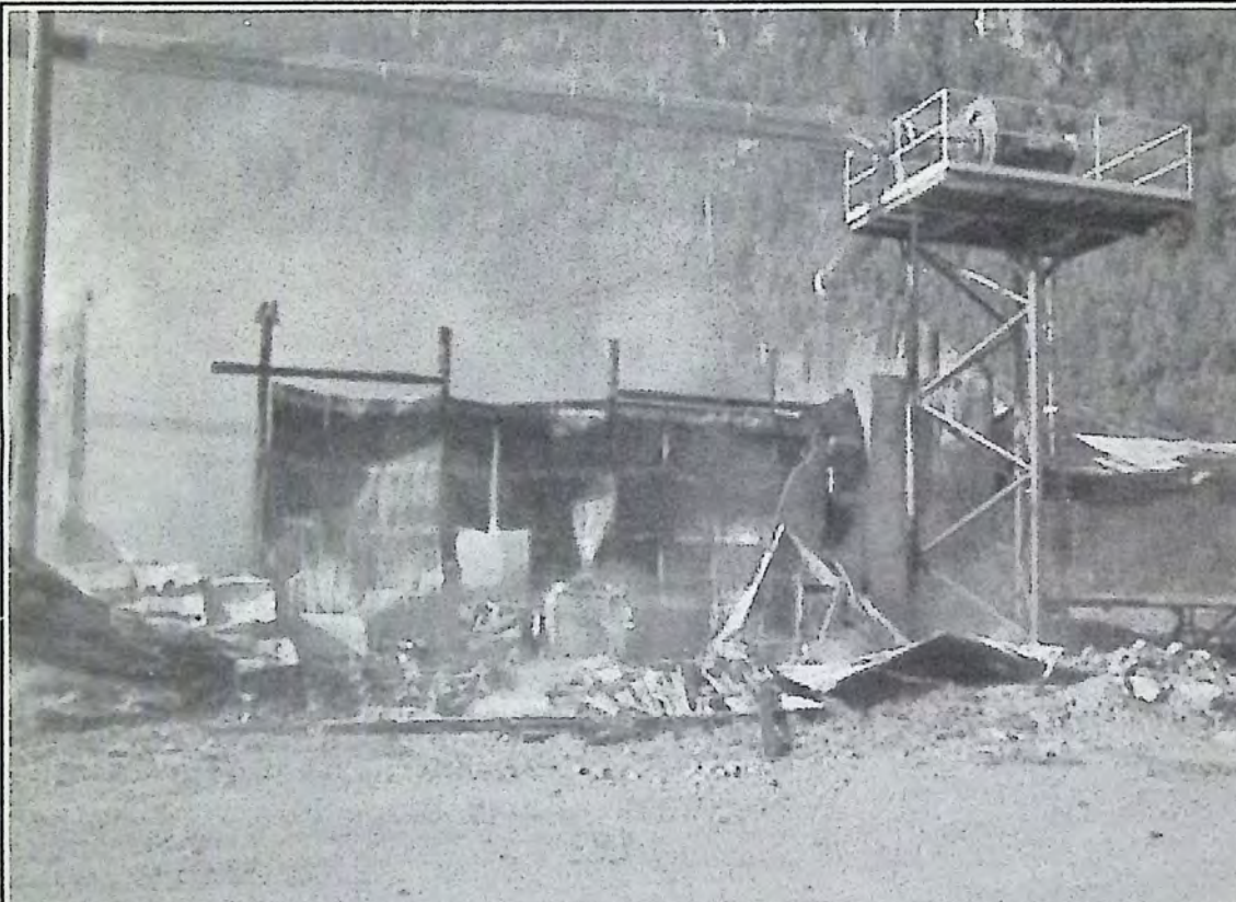
The remains of the peeler building and electrical room at PWP. - photo submitted
