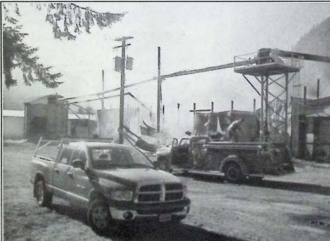
Another view of the damage at PWP. - photo submitted
