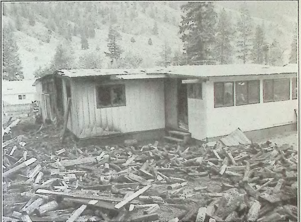
This Olalla mobile home was gutted in a fire August 21st. Photo: Alan Thom, www.OkaSimToday.com.
