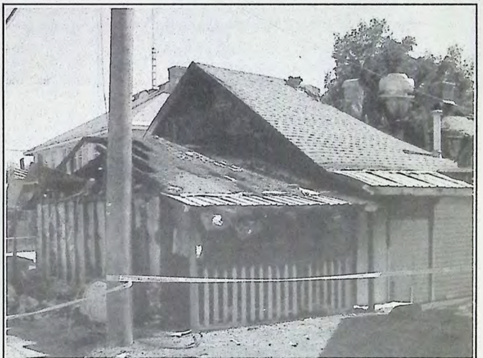
The back of the building, the kitchen area, is destroyed.*
