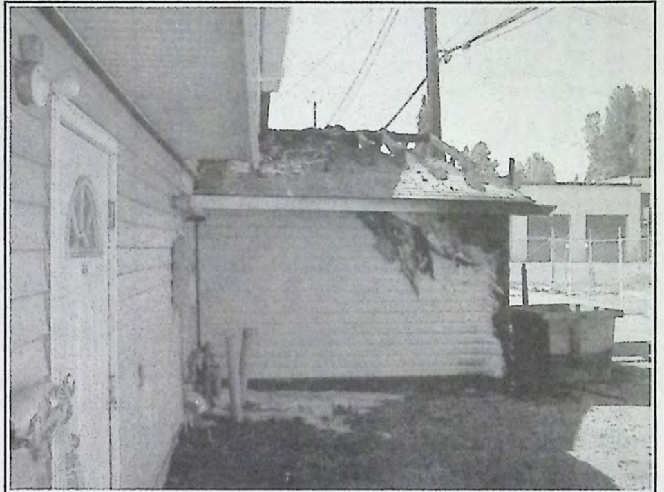
Why were there no sirens? The Fire Hall garage doors can be seen to the right.*
