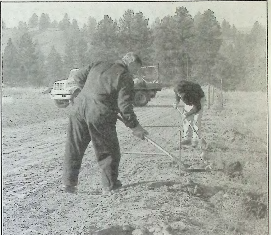
Crews worked last week on the chain link fence project at Princeton Fairgrounds. The contract continues into this week and workers say they will stay until the project is completed. *
