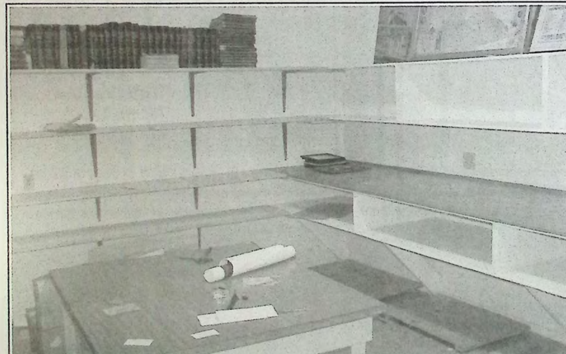
The archive room in Princeton Museum was emptied last week as work continues on the basement repairs and building renovations. *
