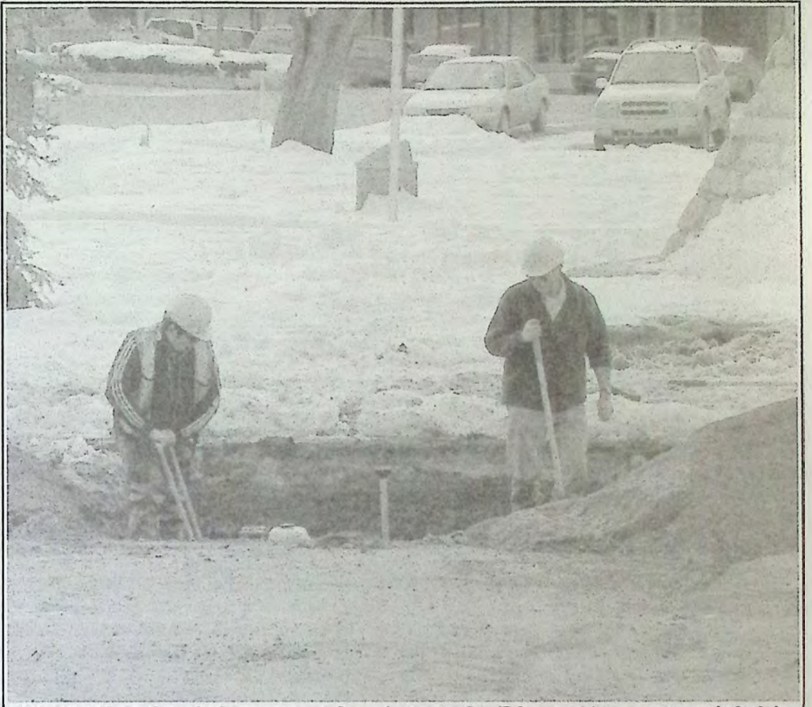
Princeton Town Crew had an unexpected repair to attend to February 21st - a water main leak in the heart of downtown forced a temporary closure of Bridge Street to allow for repairs. *
