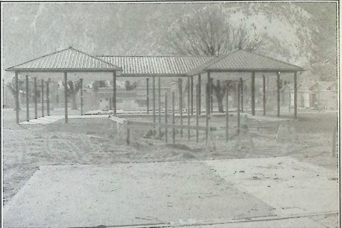
Some of the playground equipment located in Memorial Park will have to be moved to allow for the new Community Resource Centre. Crews have already removed some of the equipment. The foundation in the foreground is where the former Similkameen Country InfoCentre building sat. *
