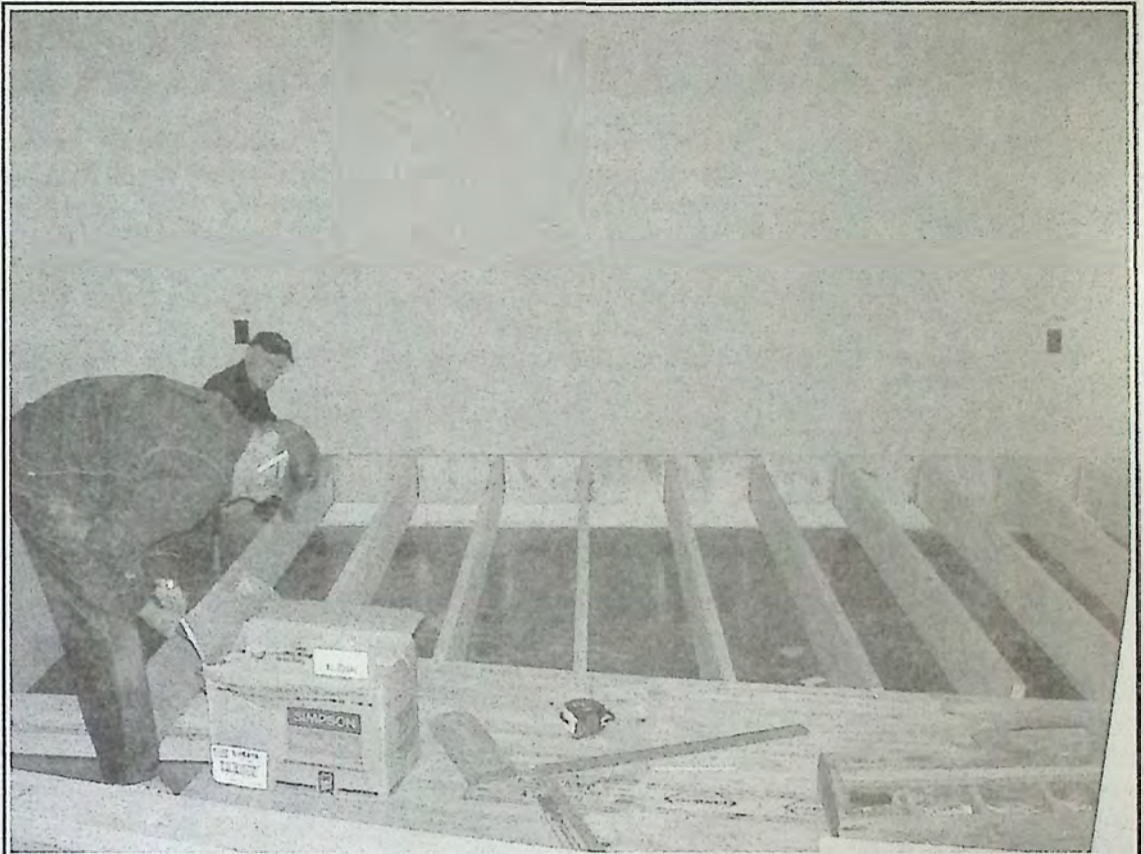
George Anderson and Lyle Hembruff have been renovating the Hedley Museum. - photo submitted
