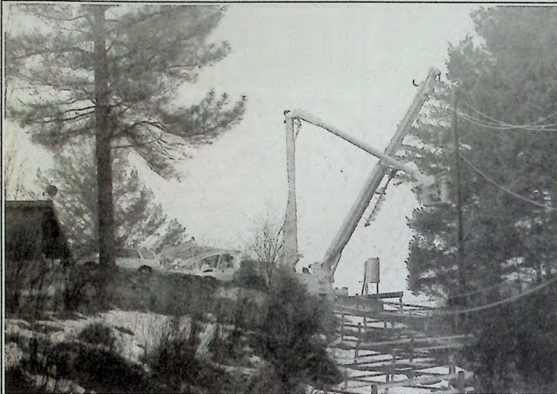
FortisBC worked all night and for most of the day March 14th to replace and repair a power pole that had been smashed in a single vehicle accident at the top of the 'zig zag' walk from First Bench to downtown. A portion of Bridge Street was without power (including the News Leader office) but crews restored it at exactly 9:00 AM to aid businesses affected by the outage. *
