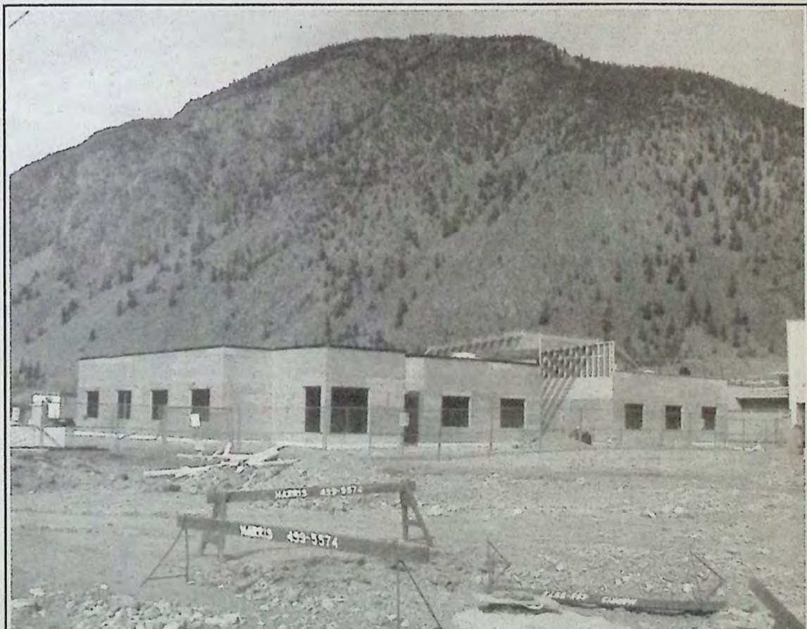
Construction on the expansion project at Orchard Haven continues to make progress in Keremeos. *
