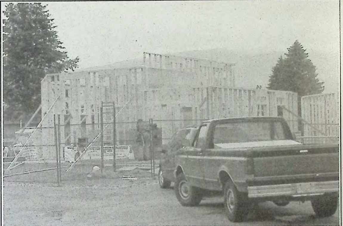
Framing went up last week on the Community Resource/Travel InfoCentre in Keremeos. Photo: Dawn Johnson
