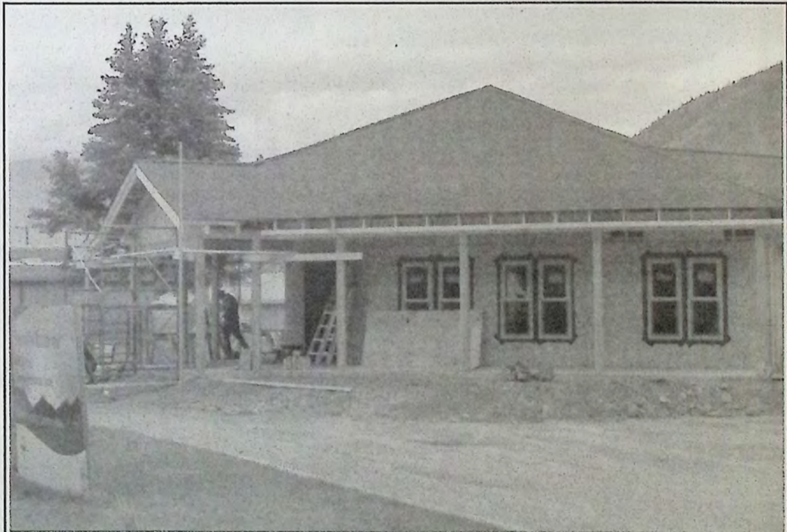
This is the new - under construction - home of Similkameen Country in Keremeos.*
