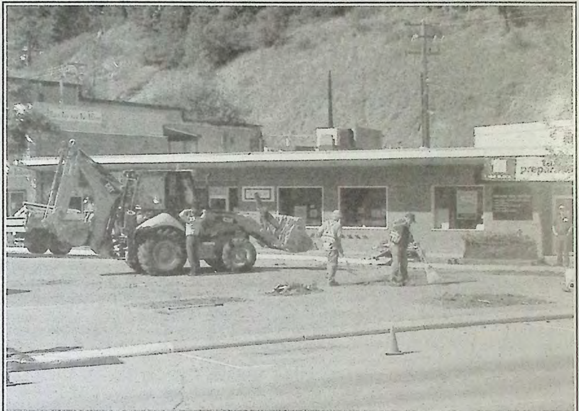
The Town Square Project started last week with the removal of planters and the curbing at Vermillion Avenue and Bridge Street. Due to high tender quotes far in excess of the money budgeted, Town Council has decided to be its own contractor to build Veterans Square. Town crew and local contractors will do the work, with Dave Woodruff acting as works manager. It is unlikely the job can be completed this year, but it could be done in two phases: the Vermillion Avenue work this fall, and the Veterans Avenue work next spring. *
