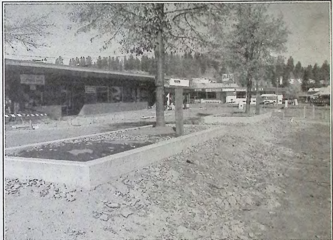
New concrete flower beds have been poured as part of the changes to be made at the Town Square. *
