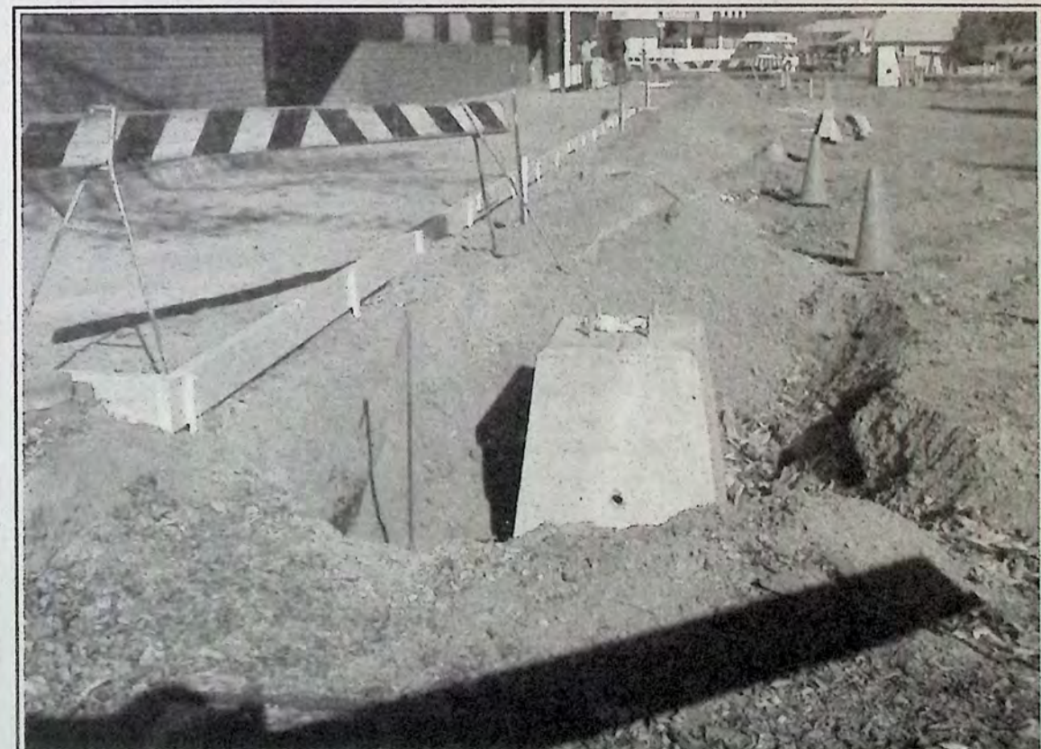
New sidewalk forms have been put in place to better define their location at the Town Square. *
