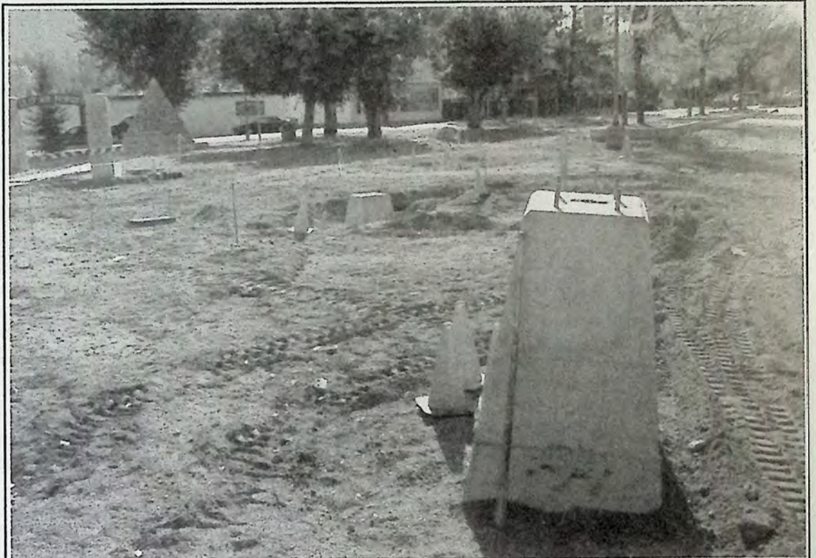
The Town Square Project continues to take shape. We wandered around the construction site last Saturday morning to see what was going on and to imagine the final outcome. *
