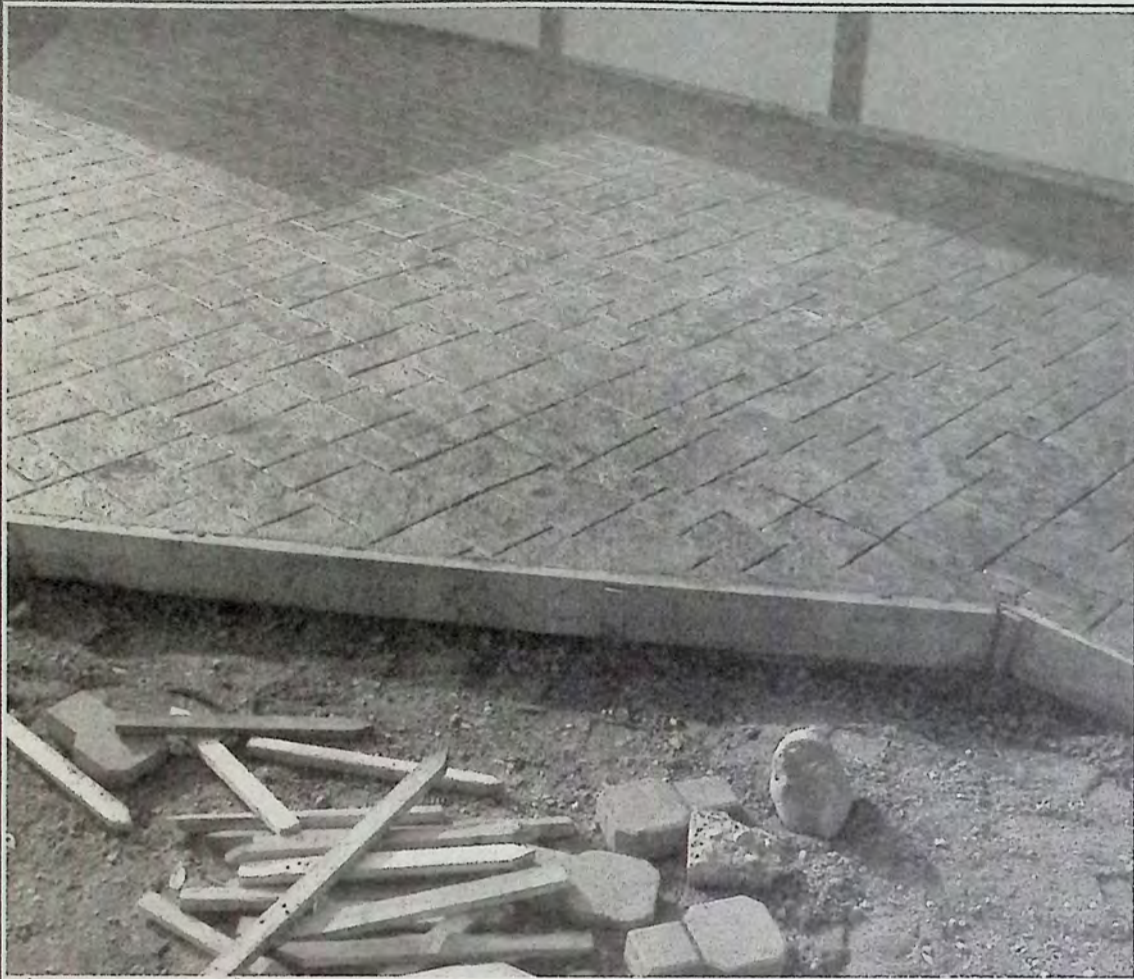
As work continued last week on the Town Square Project we managed to get this photo of a section of the new sidewalk outside Bugnuts Toys. The sidewalk is expected to be open to foot traffic soon. *
