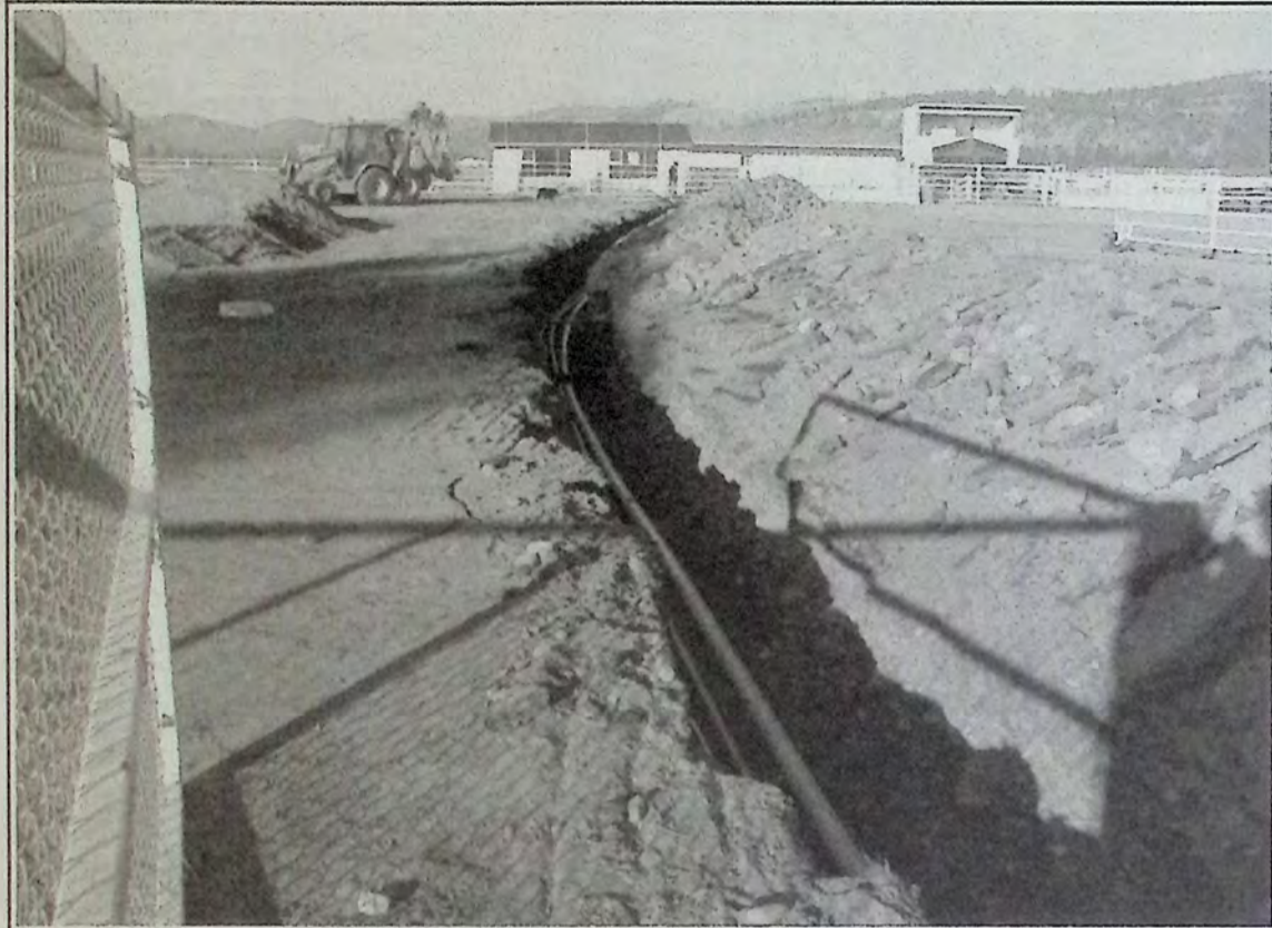
What looks like a bad case of gophers is actually work being done at Sunflower Downs to move water lines and power service underground. This is the view across the race track and into the rodeo arena. *
