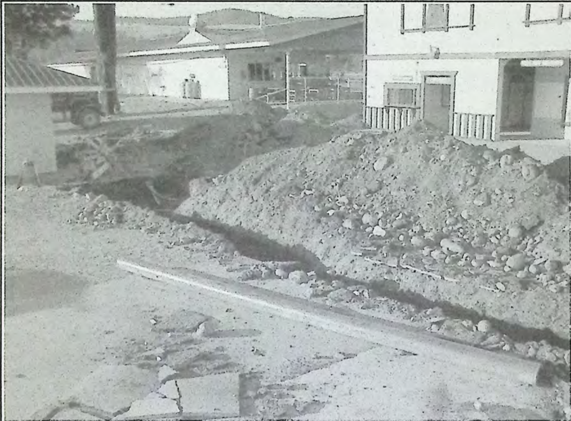
The underground water/power project last week at Princeton Fairgrounds changed the look of the facility. *
