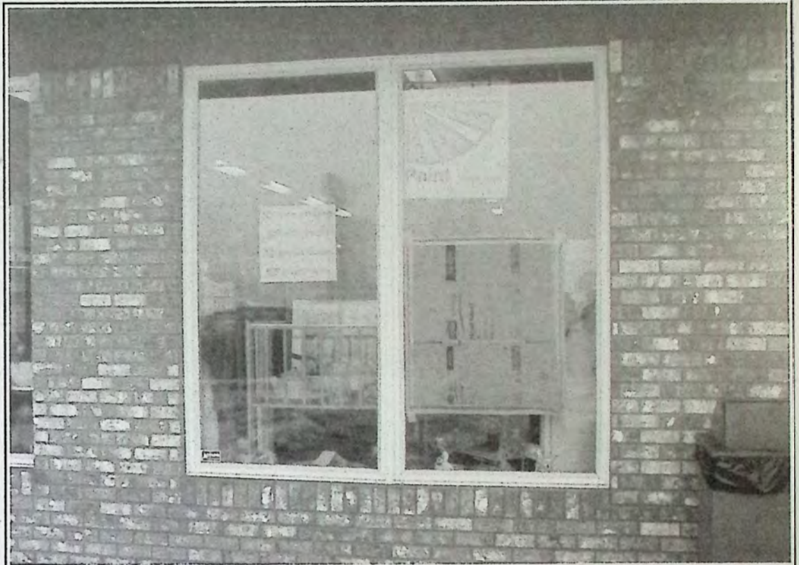
The front window at Princeton Paint & Decorating was smashed last February 3rd along with many other windows in Princeton Plaza and a couple of businesses downtown. *
