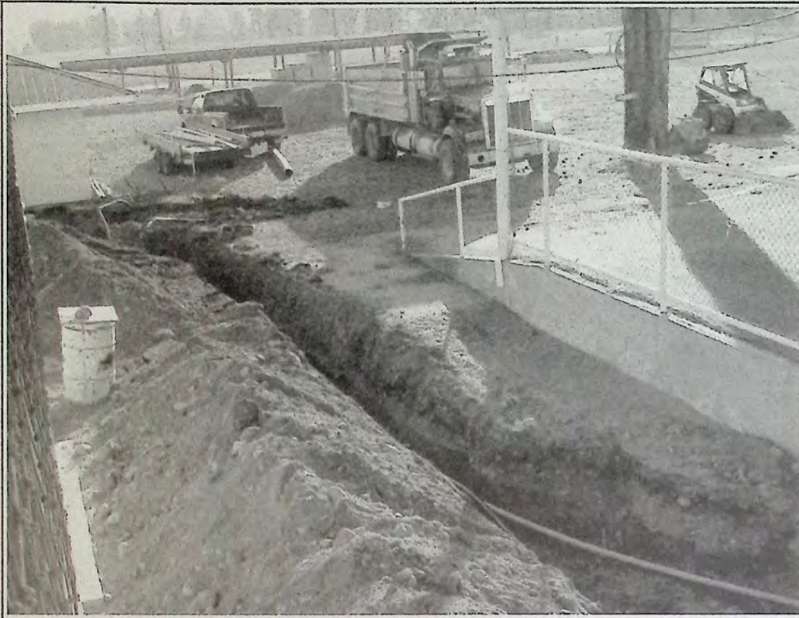
A major project at the end of 2008 at Princeton Fairgrounds saw all utility services move underground.*
