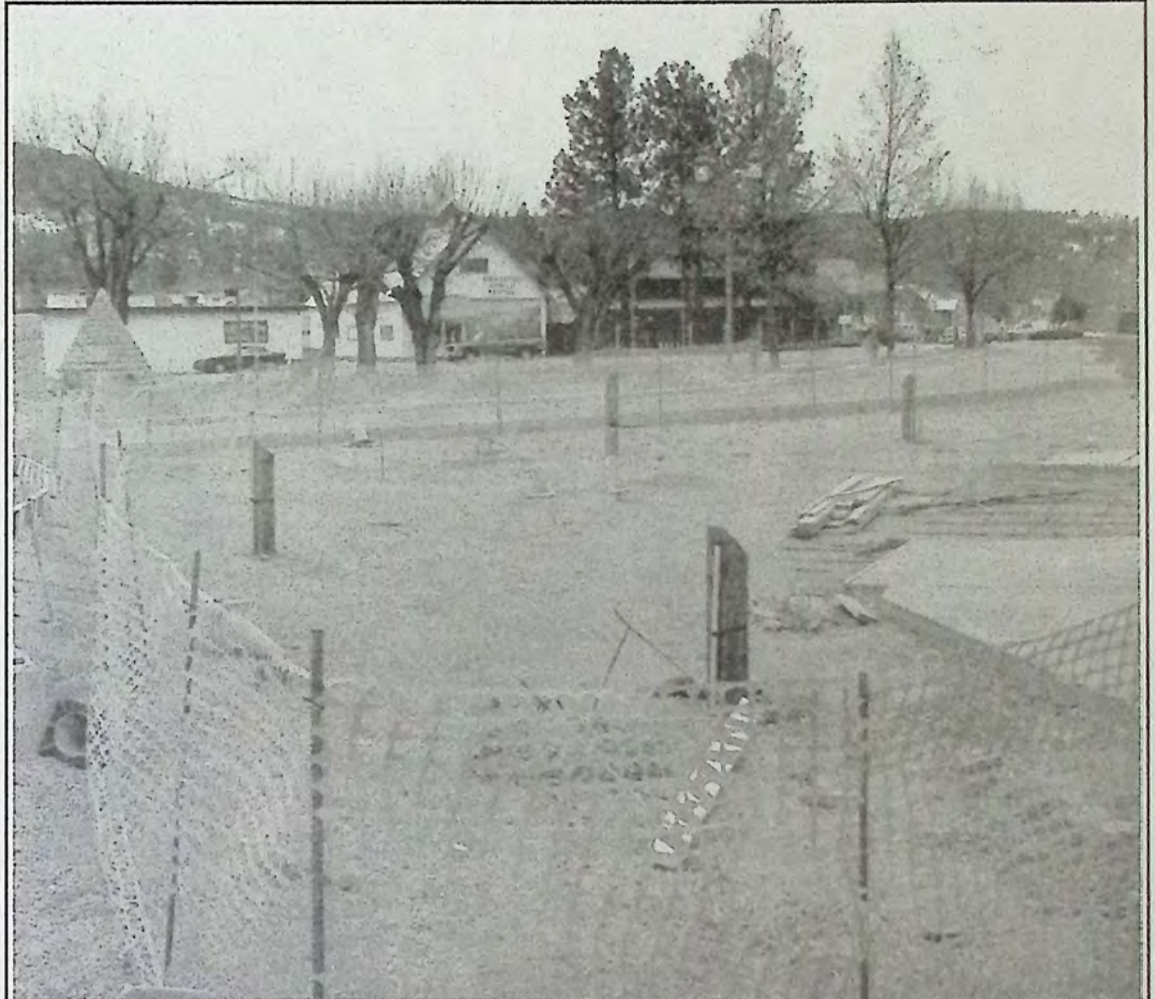
We're excited that work on the second phase of the Town Square Project will begin soon.*
