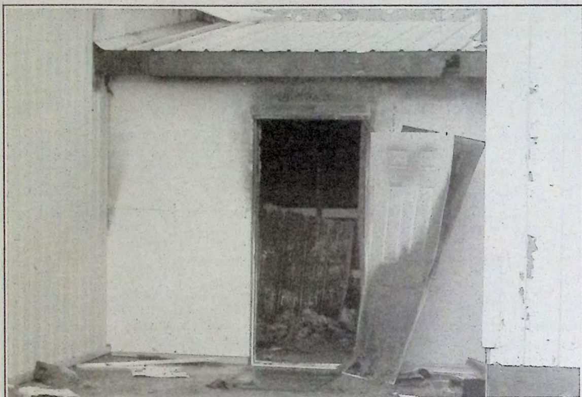
The door accessing the hallway between Princeton Arena and the Princeton Posse dressing room area hints at the extent of damage resulting from a fire early in the morning of April 6th. Photo: Brenda Engel
