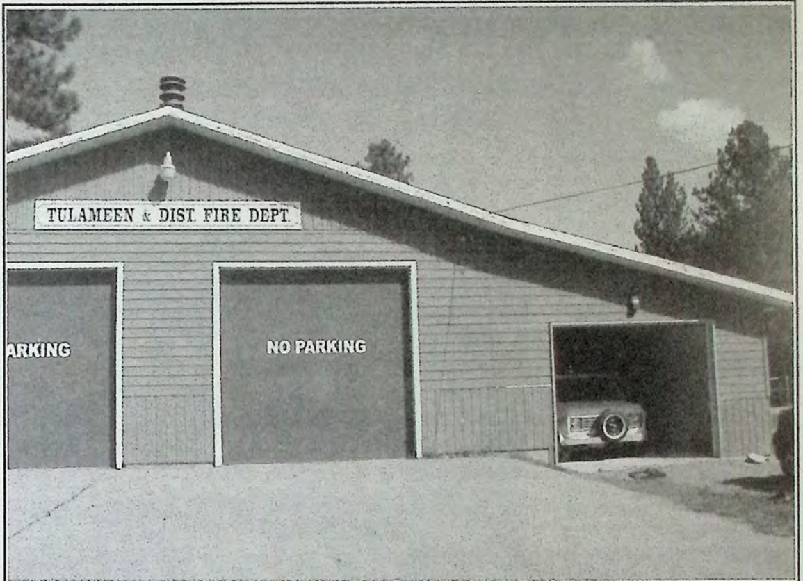
The new addition to the Tulameen Fire Hall is nearly complete. The addition (right) was built to provide a separate bay for the ambulance. Photo: Dawn Johnson
