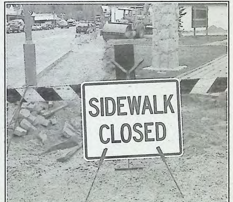
We found this sign rather funny considering the sidewalk in question is actually missing as crews continue work on the Town Square. *
