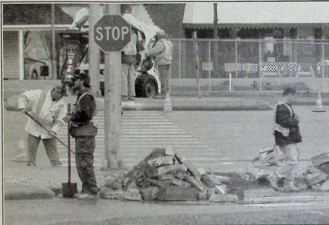
Crews worked May 14th at cutting away sections of the traffic islands at the Burton Avenue/Highway 3 intersection to improve accessibility. More work is expected at the location. Photo: Brenda Engel
