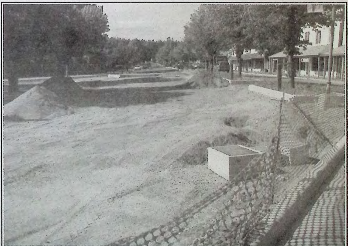
This will eventually be a large green space as part of the Town Square Project. *
