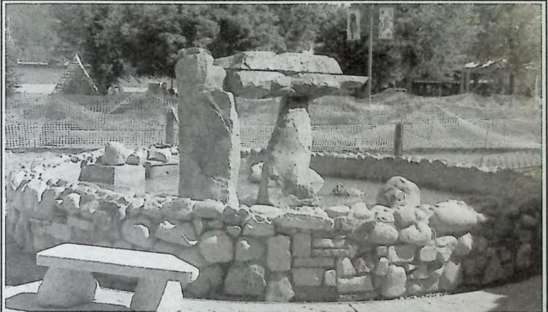
Progress continues on the Town Square Project. Last week the fountain was on for testing purposes and a short dedication ceremony. It will be a major feature of the finished project. *
