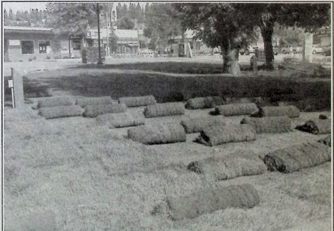
Sod went down August 17 and 18 marking the end of the Town Square Project. *
