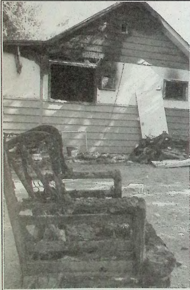
Another view of fire damage to a Cawston home August 25th. - photo and story submitted by KVFD
