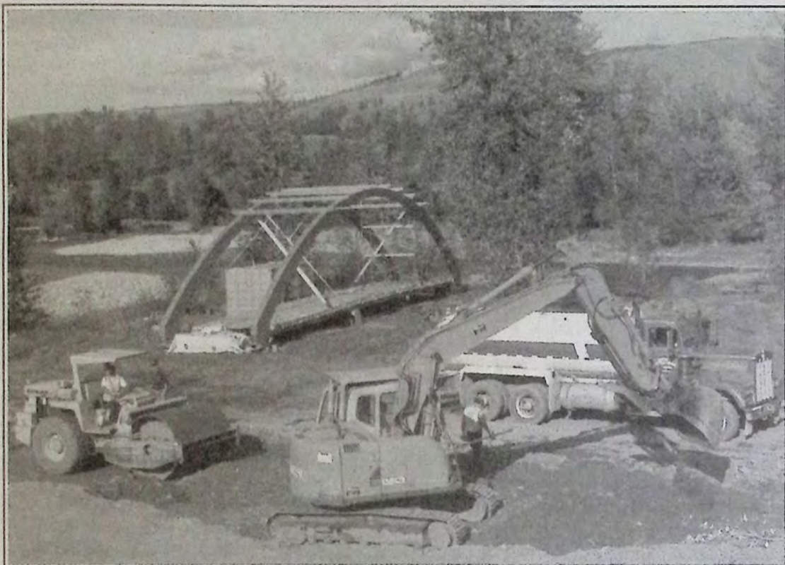
Work continues on the Bridge of Dreams linking the Trans-Canada Trail over Tulameen River. *
