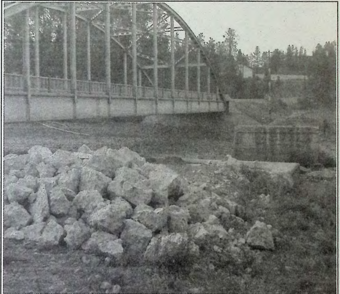
Site preparation continues this week for the Bridge of Dreams over Tulameen River at Highway 5A. *
