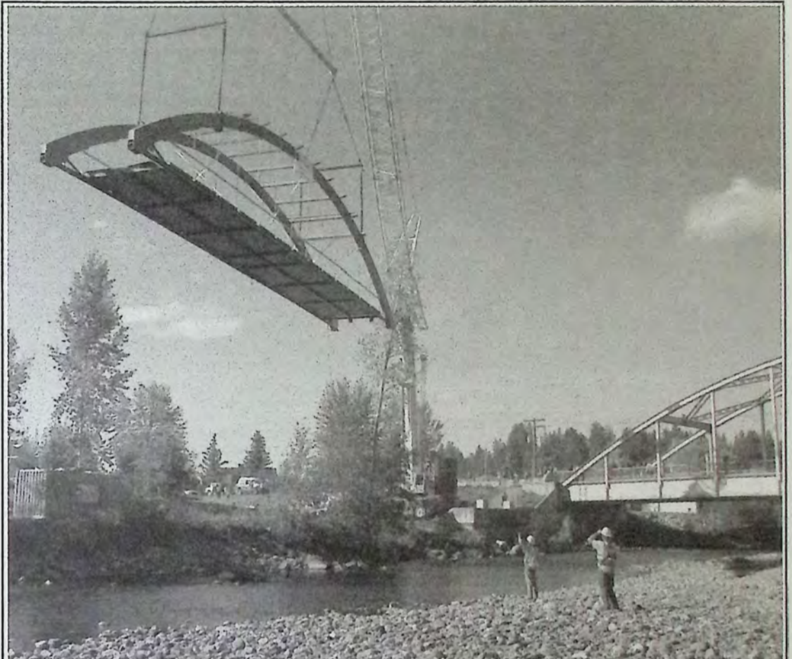
After a series of structural checks, the first part of the Bridge of Dreams was lifted into place over Tulameen River. The September 17th event turned into a huge spectator sport drawing many onlookers. *
