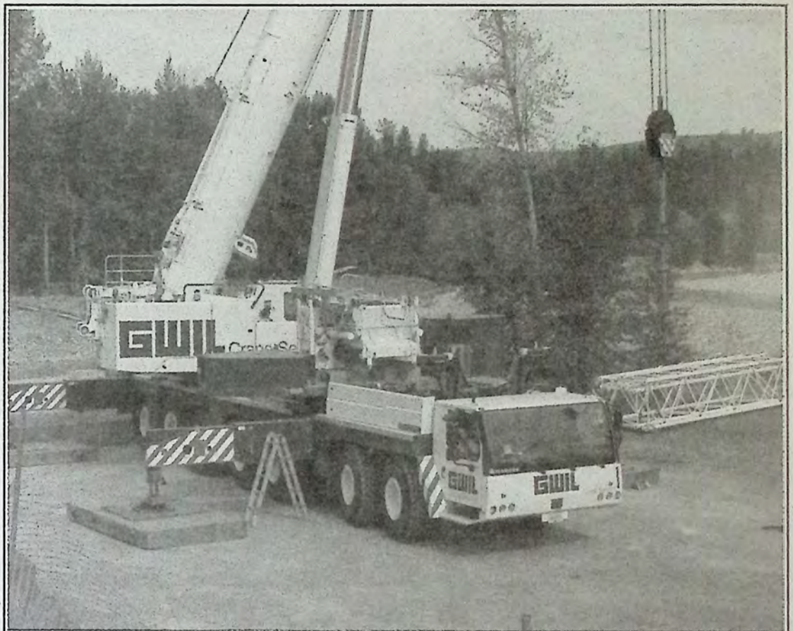
It came to town in pieces and will leave the same way. One of the largest cranes in western Canada. *
