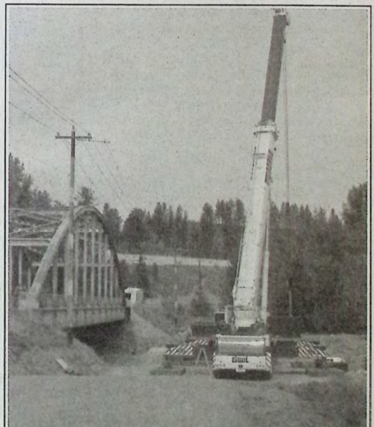
This photo only hints at the size of the crane that moved into position September 15th along the Trans-Canada Trail for placement of the Bridge of Dreams across Tulameen River. *
