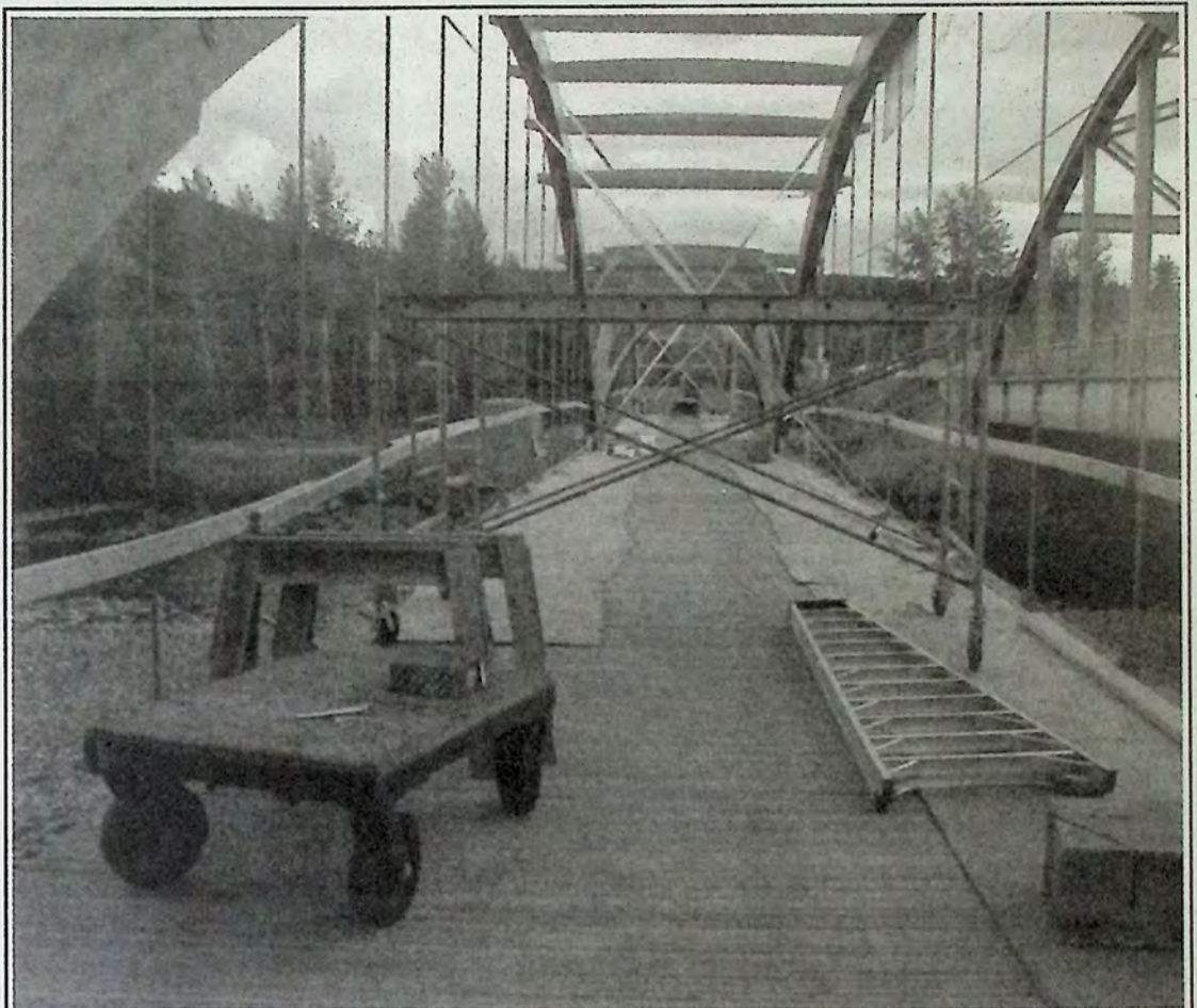
A look across the Bridge of Dreams at Tulameen River. Crews continue to work on the project. *
