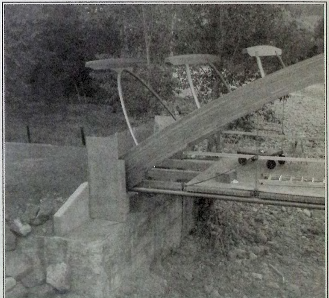
The Trans-Canada Trail grade now meets the Bridge of Dreams on one side. *
