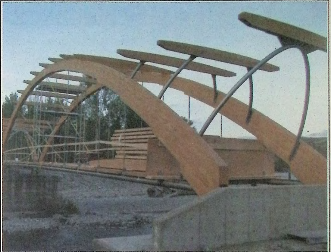
An interesting view of the Bridge of Dreams across Tulameen River shows some of the additional detailing that has been installed as the project continues to get closer to completion. *
