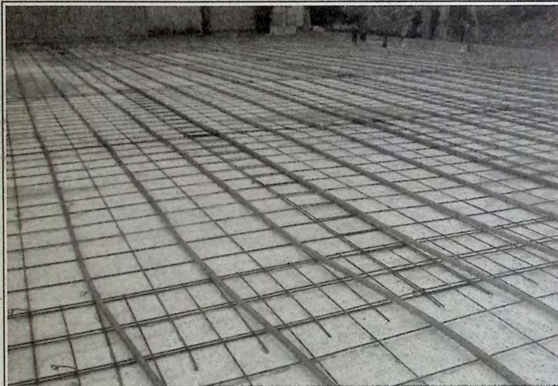
The foundation was back filled last week with floor heating plotted out. *
