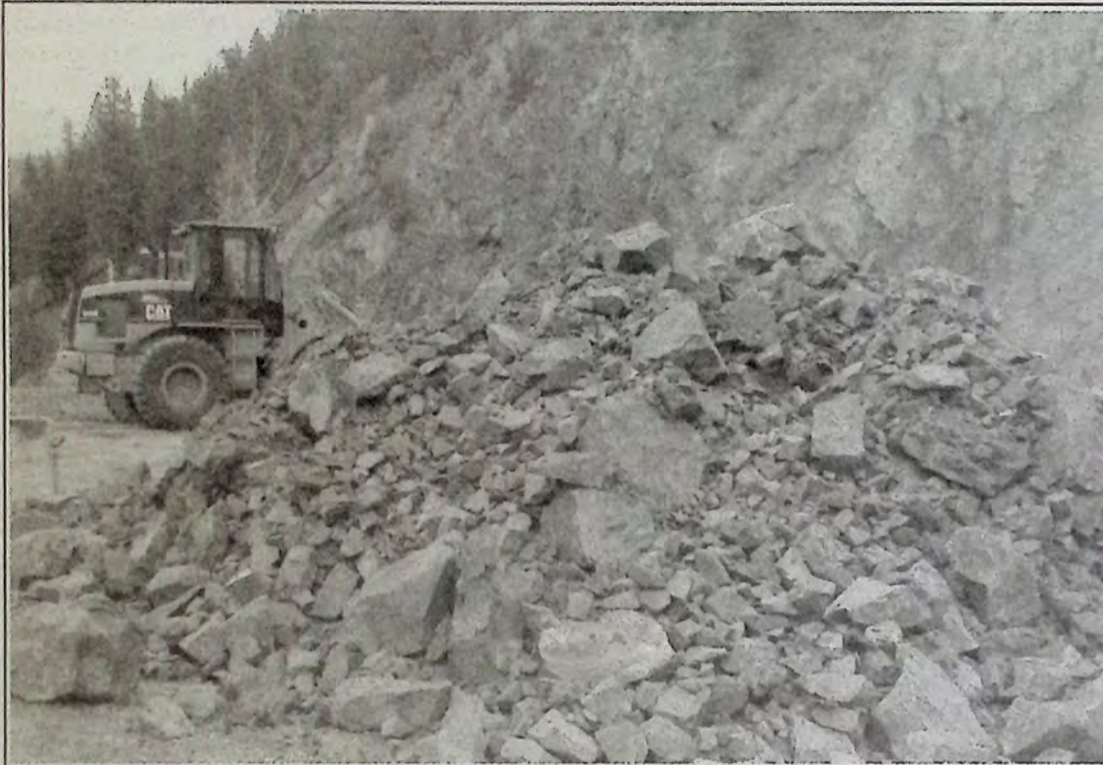
A rock slide on Tulameen Road near the Red Bluffs closed the route to all traffic for a period of time October 21st. Crews had it cleared by early afternoon. Photo: Brenda Engel
